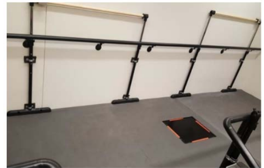
FootSTEPS installed in elevated walkway at Univ. of North Texas Health Science Center (courtesy of Dr. Metin Yavuz).
